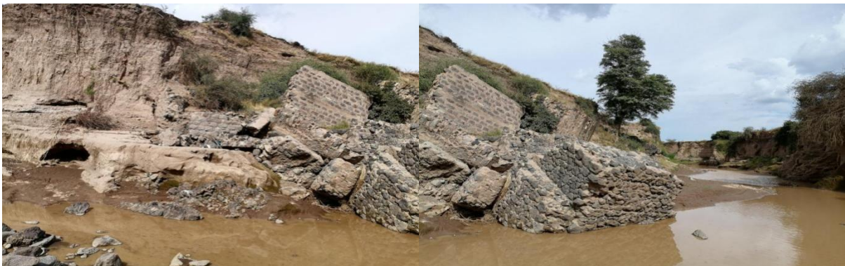
FIGURE 1.1: FAILED ABUTMENT OF THE OLD ETHIO – DJIBOUTI RAILWAY BRIDGE DUE TO SOIL EROSION
