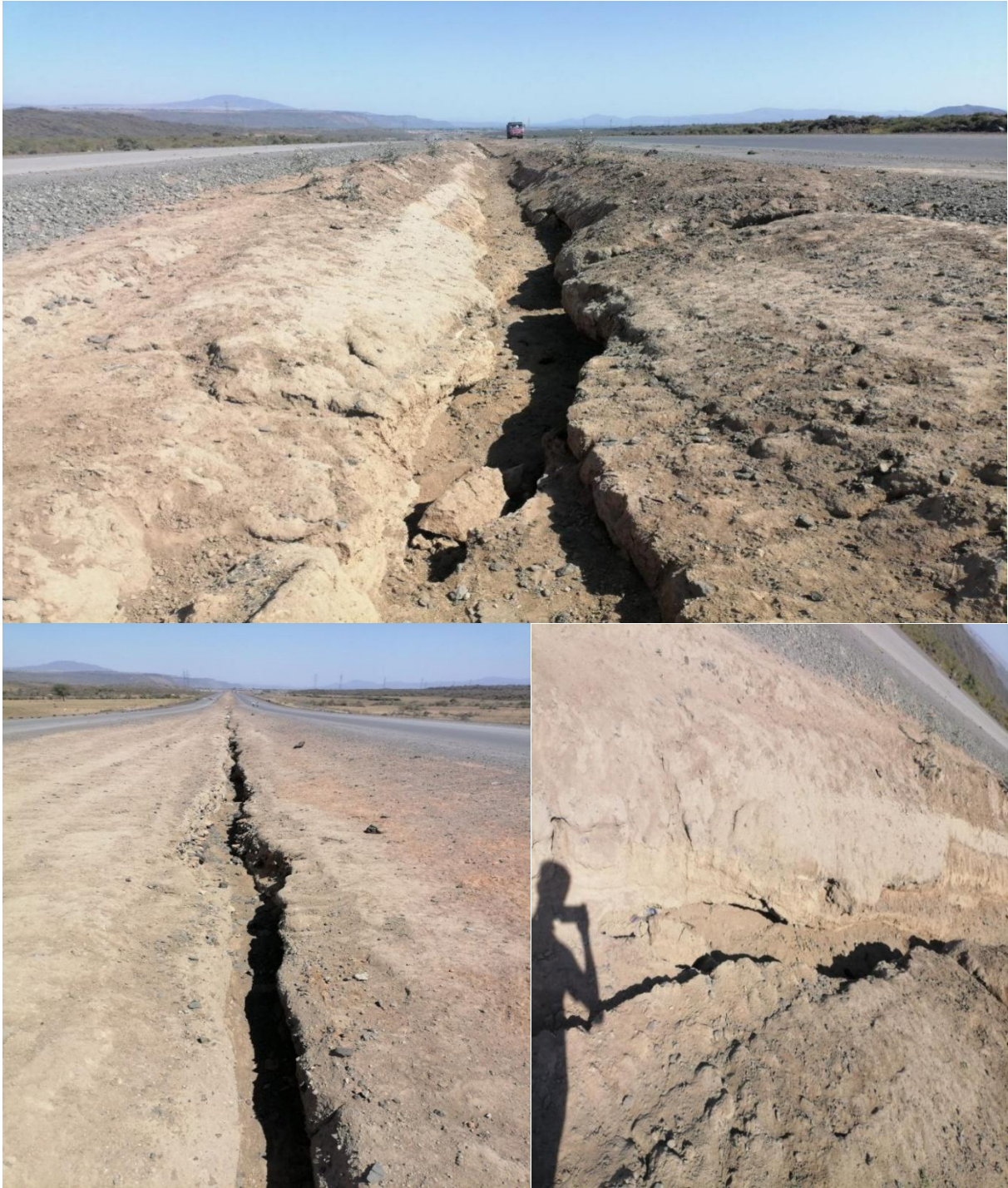
FIGURE 4.5: EROSION PATTERNS ON MEDIAN EARTH DITCHES OF THE EXPRESSWAY
