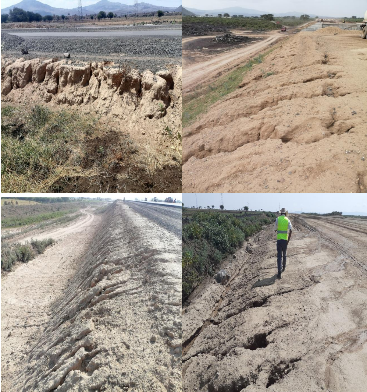
FIGURE 4.1: PIPING EROSION ON THE EMBANKMENT OF THE EXPRESSWAY
