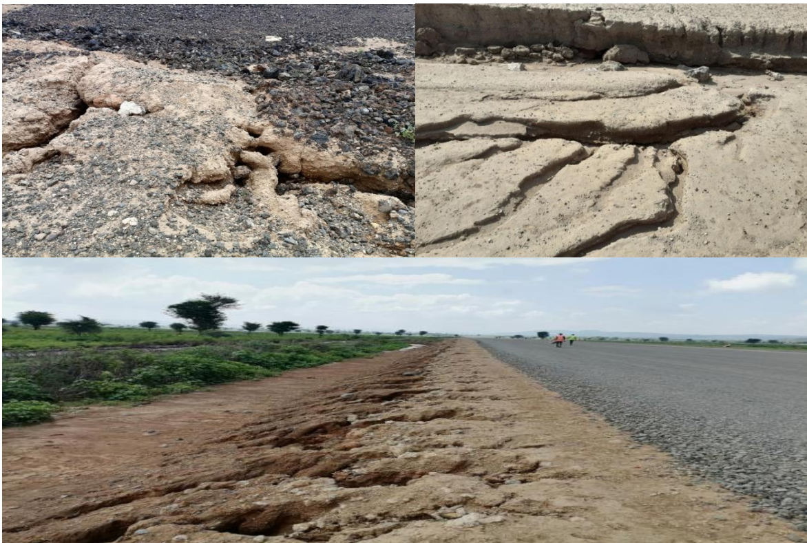
FIGURE 4.4: EROSION PATTERNS ON THE SOFT SHOULDERS OF THE EXPRESSWAY
