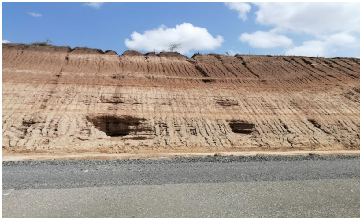
FIGURE 1.3: ERODED CUT SLOPE FACES AT ADAMA – KM 60 EXPRESSWAY PROJECT
