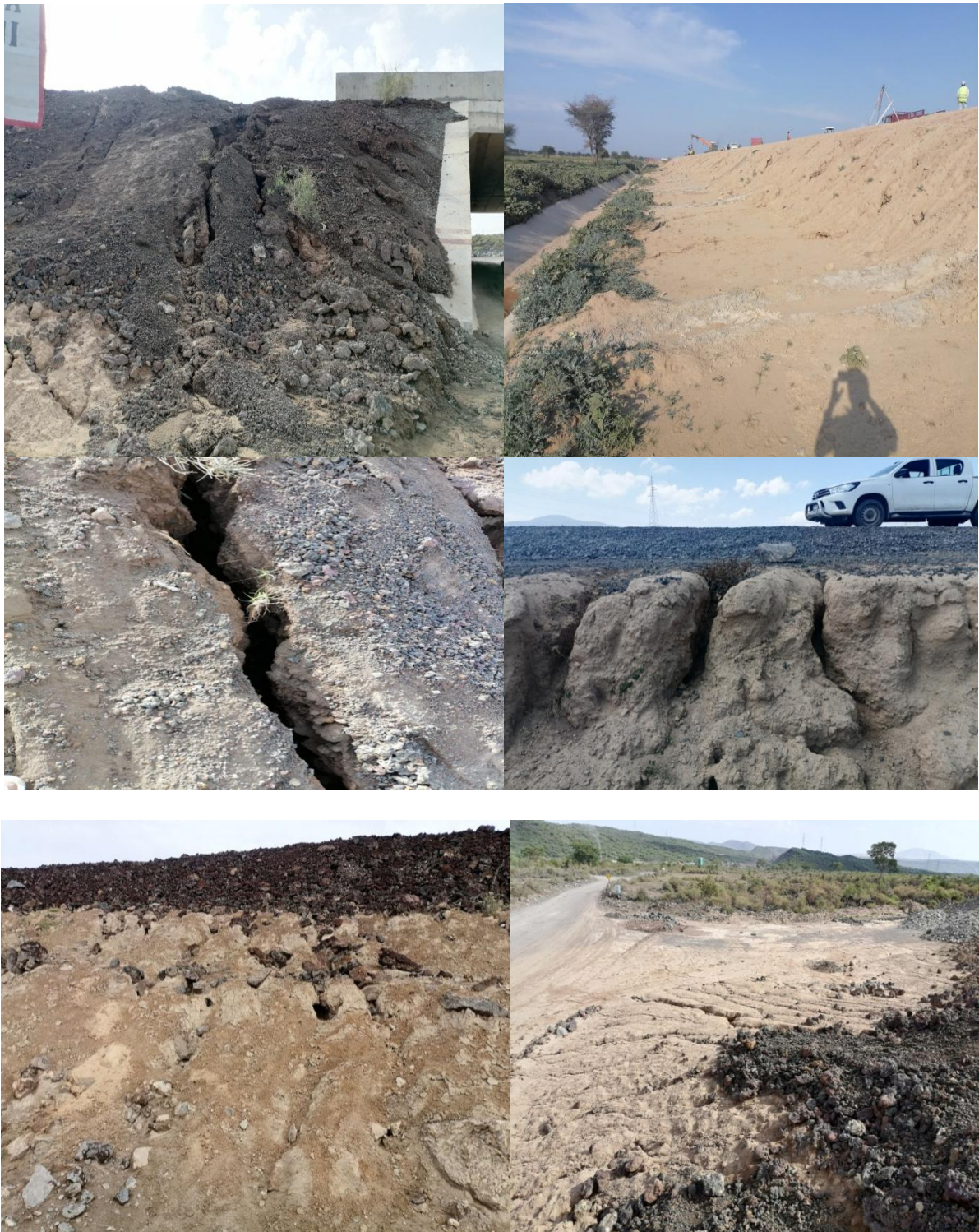
FIGURE 4.2: DIFFERENT TYPES OF EROSION PATTERNS ON EMBANKMENT SLOPS OF ADAMA-KM60 EXPRESSWAY PROJECT
