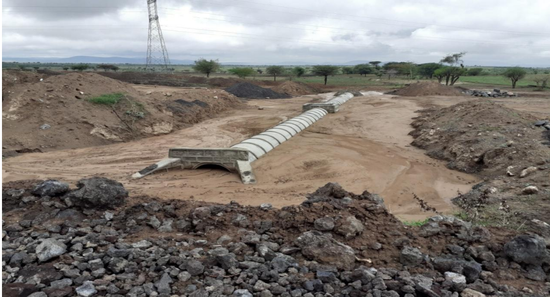
FIGURE 4.7: CLOGGED PIPE CULVERT DUE TO SOIL SEDIMENT AT ADAMA-KM 60 EXPRESSWAY PROJECT
