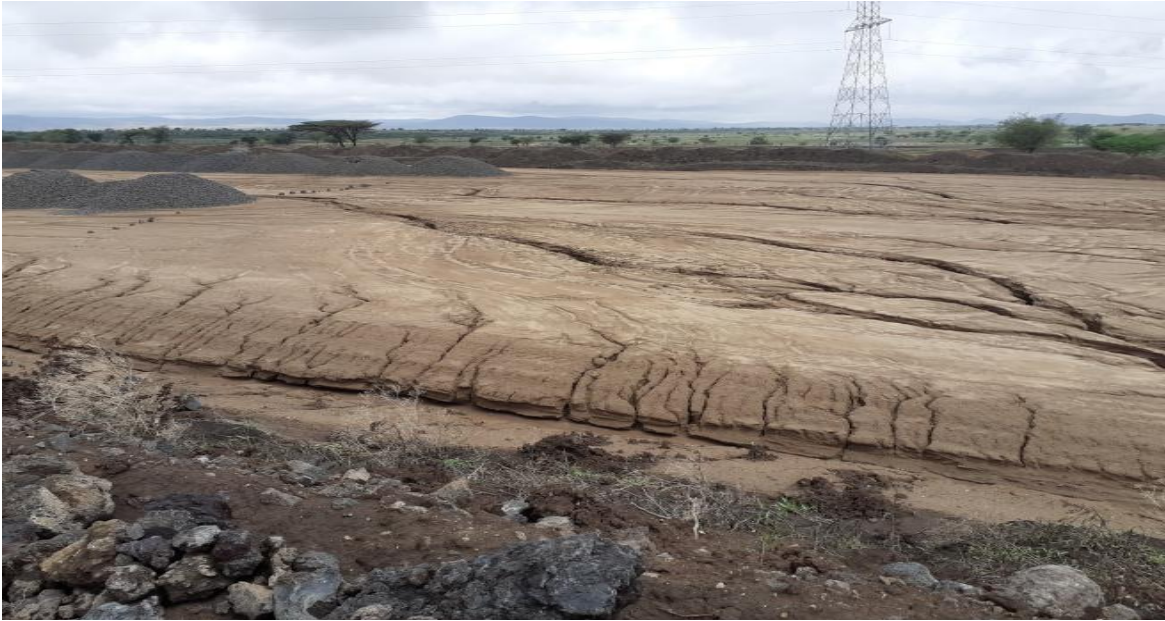
FIGURE 1.2: SOIL EROSION ON CONSTRUCTED CAPPING LAYER AND SOFT SHOULDER OF THE EXPRESSWAY
