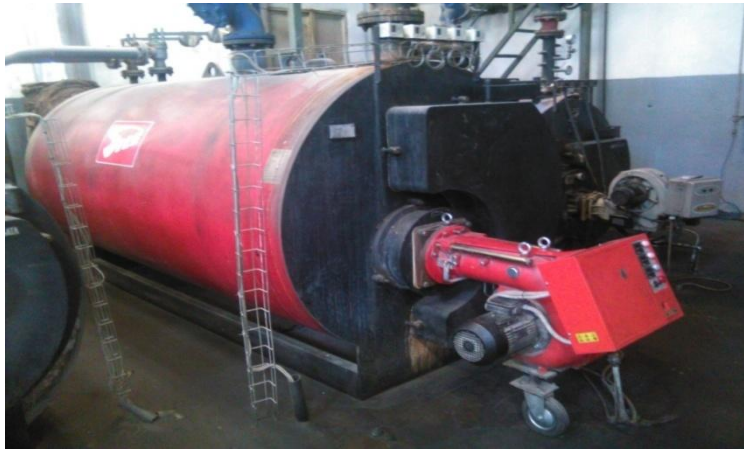
Figure: 5.1. Boiler used at the factory.
