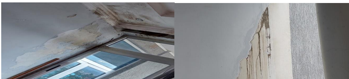
Figure 8: Dampness problem of the building
