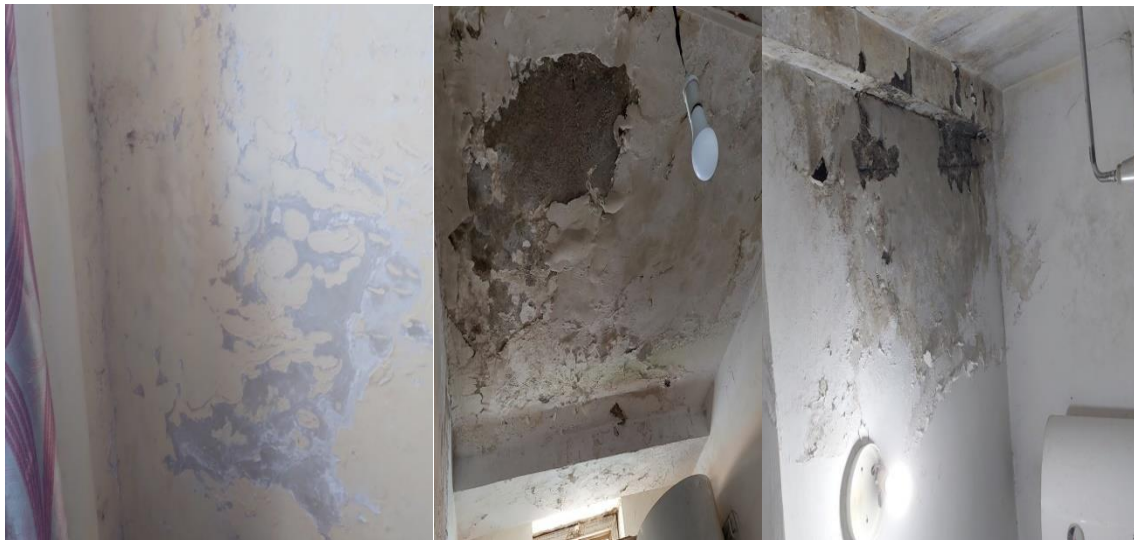
Figure 31:-Dampness of the building in toilet
