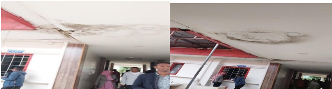
Figure 16:- Dampness exist in the buildings
