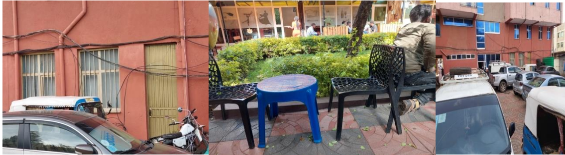
Figure 30: Rainwater through downpipe to main drainage line (Left), Ground level garden at the back of buildings and Terrazzo paved parking area at the back of the building
