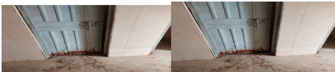
Figure 22: Dampness of the building around the toilet.
