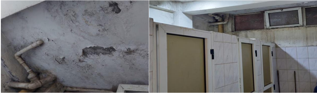
Figure 28: Dampness in the building around the toilet
