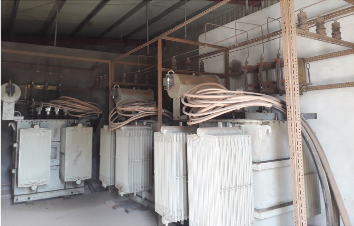
Figure 3.4: Partial view of Adama Spinning Factory power house.
