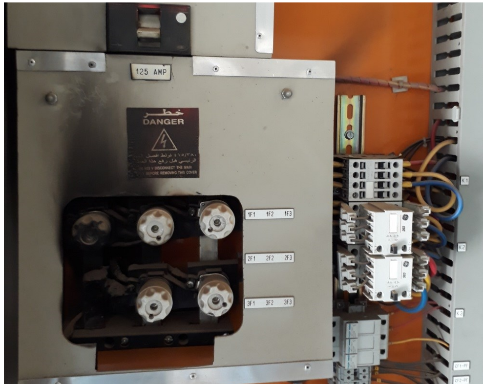
Figure 3.7: Damaged part due a sudden fire inside CMDDB-1 board.
