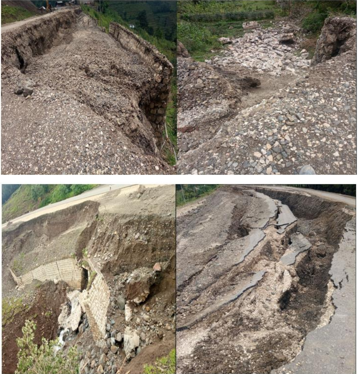
Figure 7-1 Qune-Bedesa Road section failure in July 2024 which needs Further explorations.
