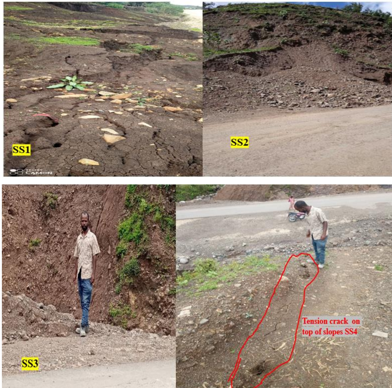
Figure 3-7 Some of visible sign of slope failures during field survey.
