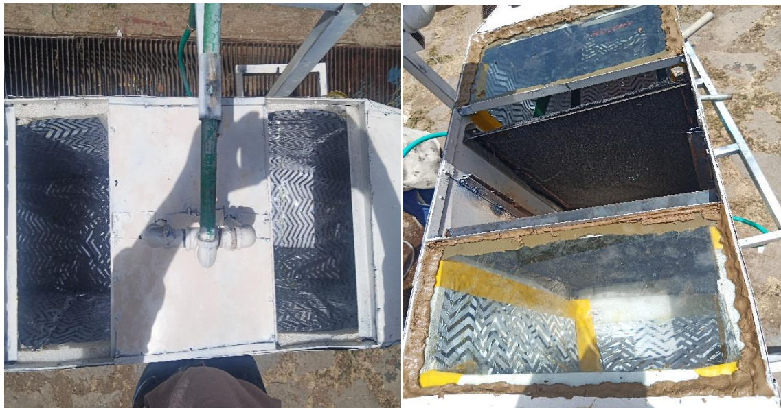
Figure 5. 3: Air filtration chamber
