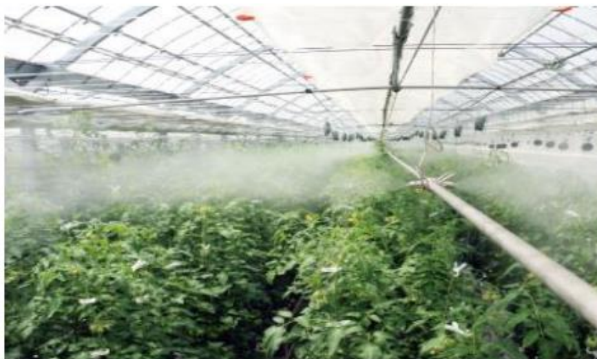
Figure: 2.14. Fogging systems for cooling a greenhouse (Kidist, 2021).
