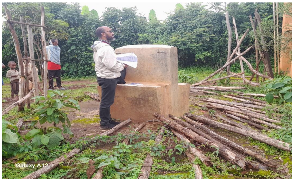
Appendix 18. Damaged water point fencing in Boyna Kare Village
