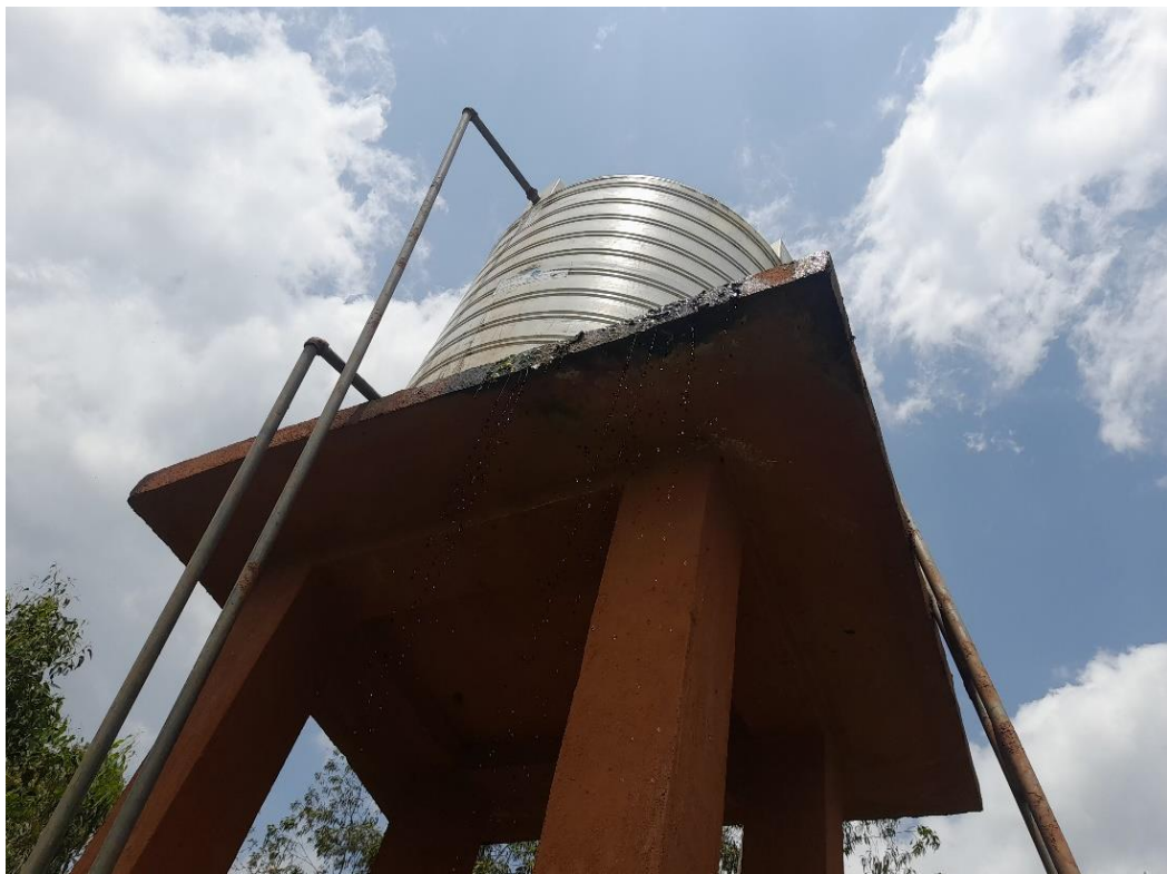
Appendix 17. Reservoir leakage problem in Mante Village, Dubo Kebele
