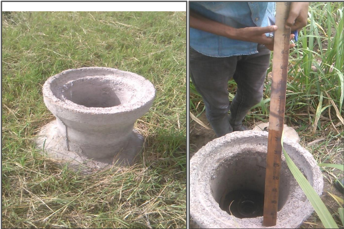
Figure 3.8: Installed Piezometer at the Field 50
