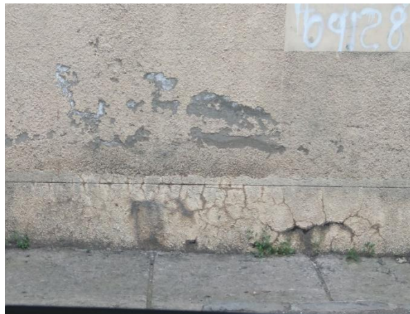
Figure 7-8 Cracks on grade beam
