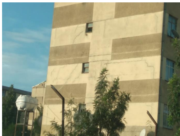
Figure 7-10 Crack on wall
