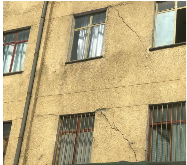
Figure 7-14 Major crack on wall
