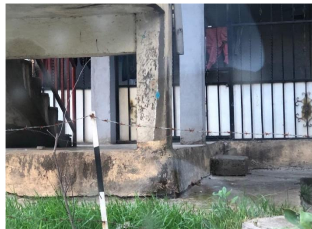
Figure 7-16 Cracks on grade beam and wall
