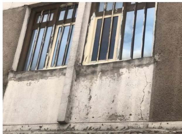
Figure 7-15 Cracks on grade beam and wall
