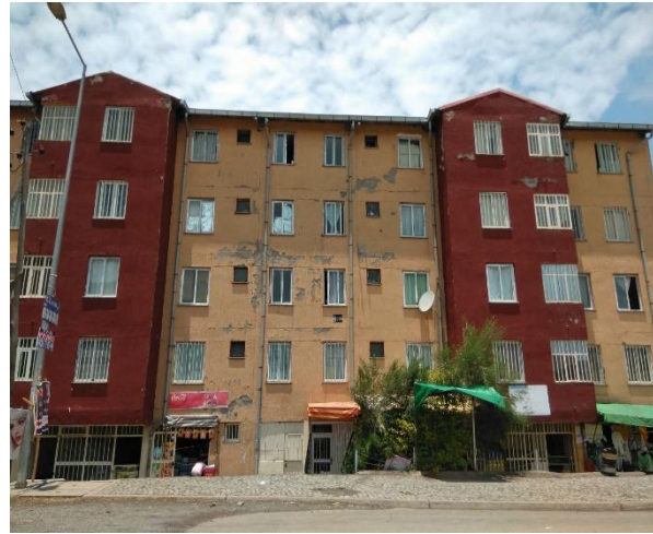
Figure 7-7 Peeled wall paint
