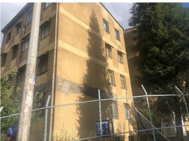
Figure 7-12 Poorly maintained beam
