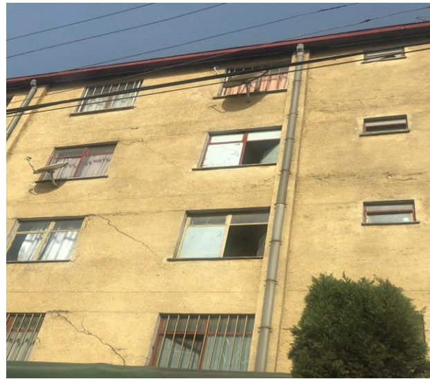
Figure 7-13 Major crack on wall
