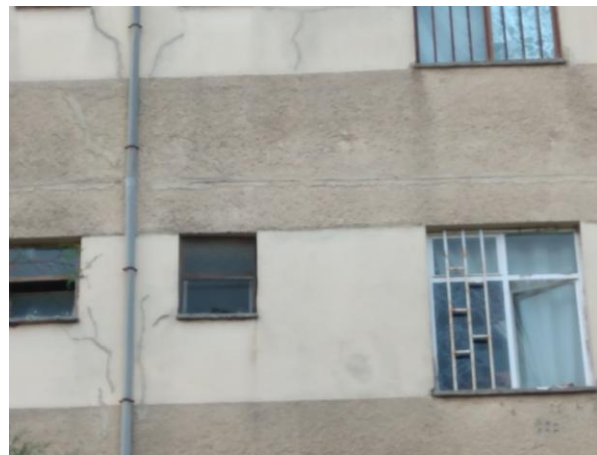
Figure 7-9 Cracks on wall
