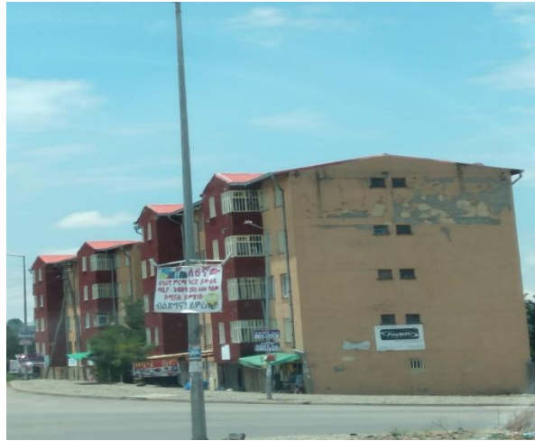
Figure 7-6 Peeled wall paint
