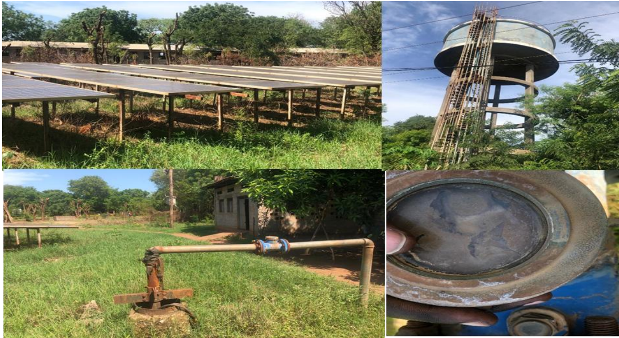
Figure 3. 2: MoWE SPWPS Components at Pinyudo High School Site
