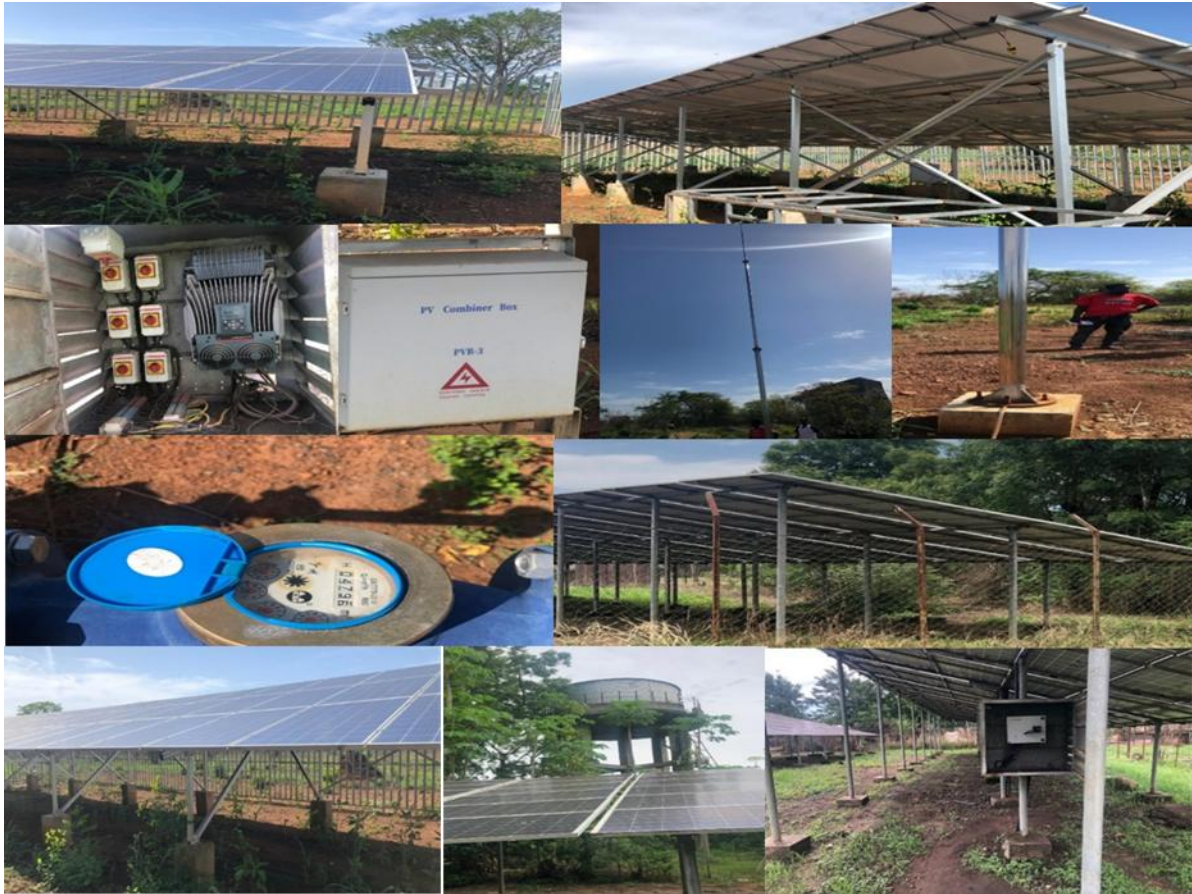
Figure 3. 4: Grundfos SPWPS Related Works at Pinyudo Town
