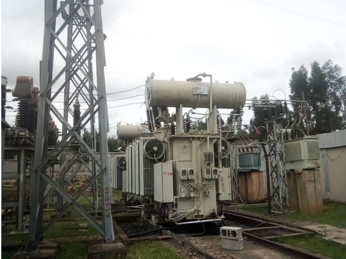
Fig. 1.1: Overview of Fiche Substation
