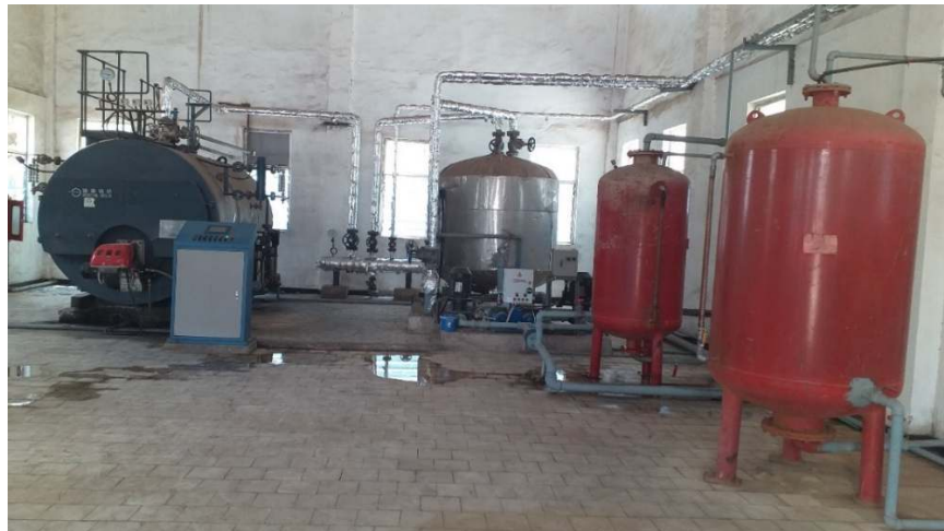
Figure 3.2. Installed diesel fuel steam generation of AHMC new building
