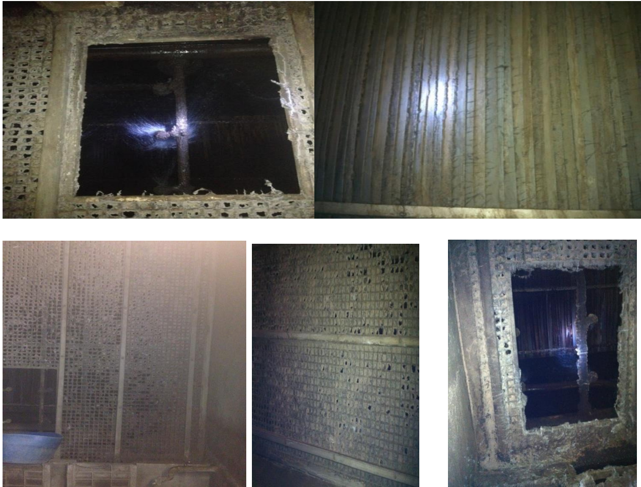
Figure.4. 13.Pictures of present condition of humidification plants
