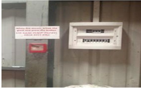
Figure.4. 10.power distribution circuit Breaker
