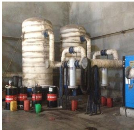
Figure.4. 14.Compressors and compressed air distribution system
