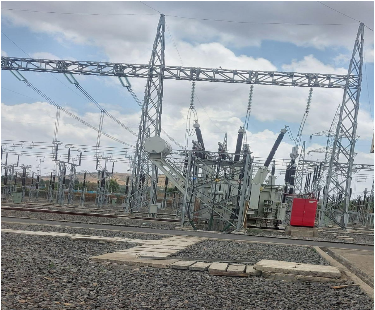
Figure 1.2 Overview of the Mojo New distribution substation taken during a site visit
